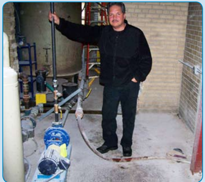
Santos Flores next to the trouble-free Griswold 811 ANSI Series centrifugal pump in a cooling application.
