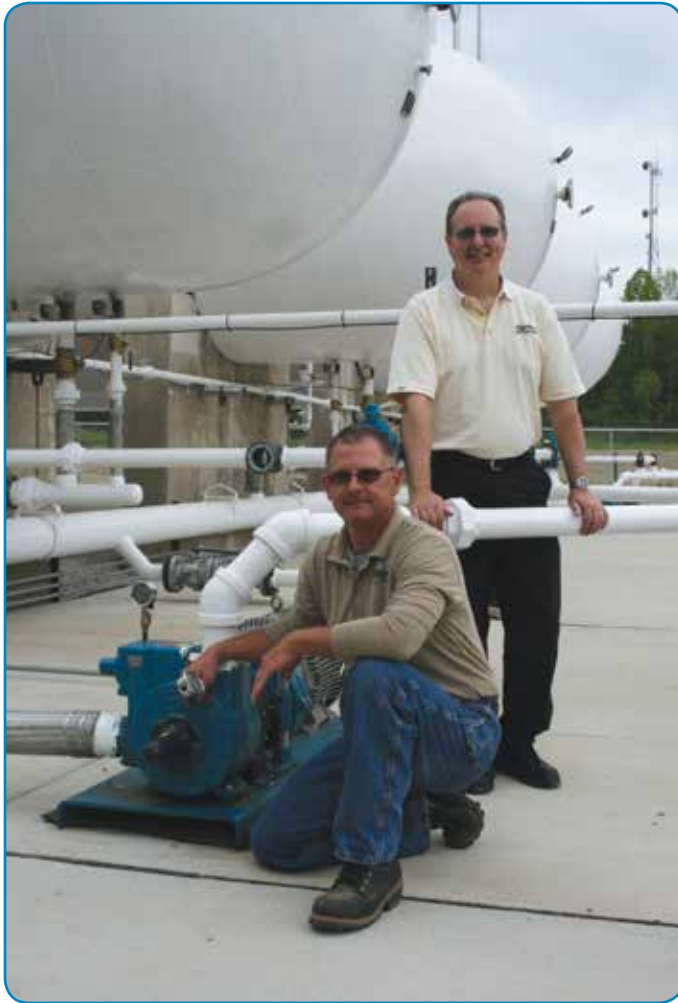
Scott Tonkin, front, Operations Manager for Altogas' Red Arrow Transfer Terminal, and Jim Becker, Blackmer®/PSG® Regional Manager, have been infinitely pleased with the capability of Blackmer's LGL Series Sliding Vane Pumps to meet the unique flow-rate needs of the new facility.
